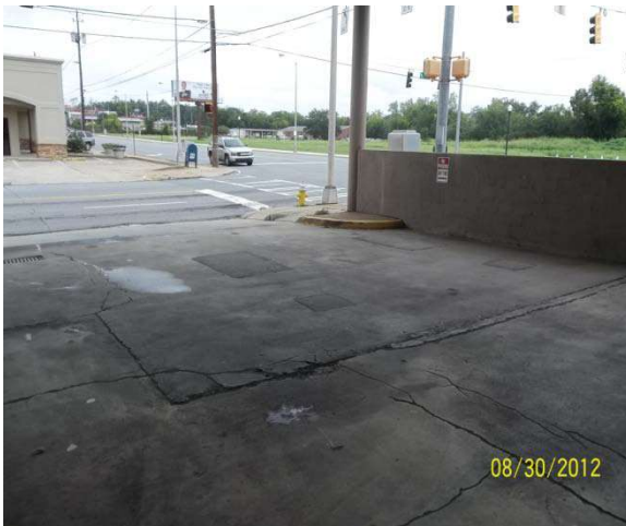
Photograph #15 View of location of closed in ground storage tanks in the northern portion of the subject site
