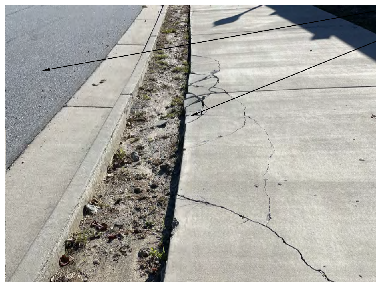
FIFTH AVE WEST DAMAGE TO EXISTING CONCRETE WALKWAYS
