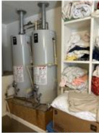
Mech Room - water heaters
