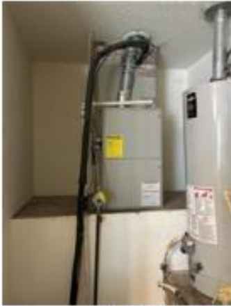
Mech. Room - heating system
