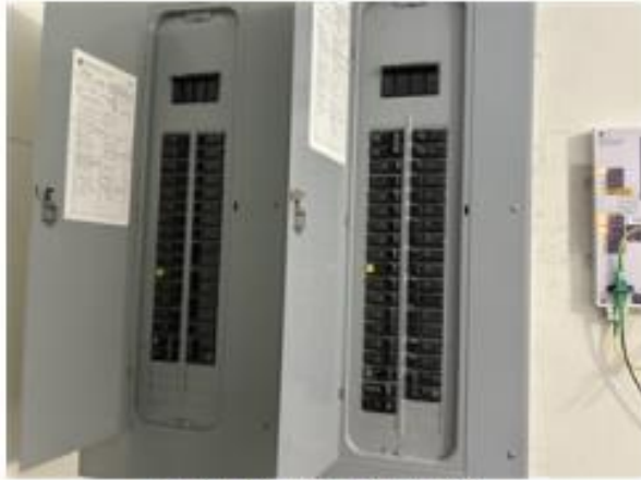
Mech.Room- electrical system
